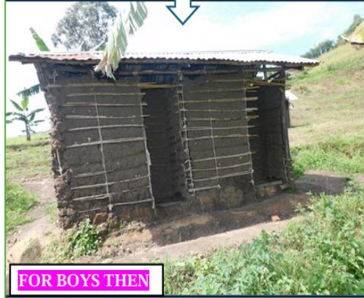
SANITATION FACILITIES BEFORE
